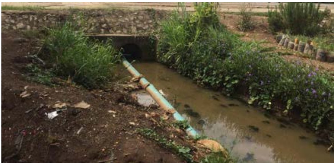
Picture 2-12: Sewer network along Ant Malaria Drainage System
