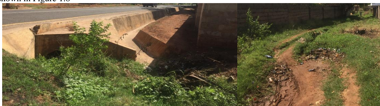
Figure 1.6 : Existing Drainage System at Baracuda along Modeco Road
